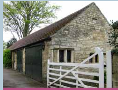
Garaging associated with ‘Box Trees’. An area of yellow stone above the right hand window suggests an opening has been filled. The date stone is set above this.
